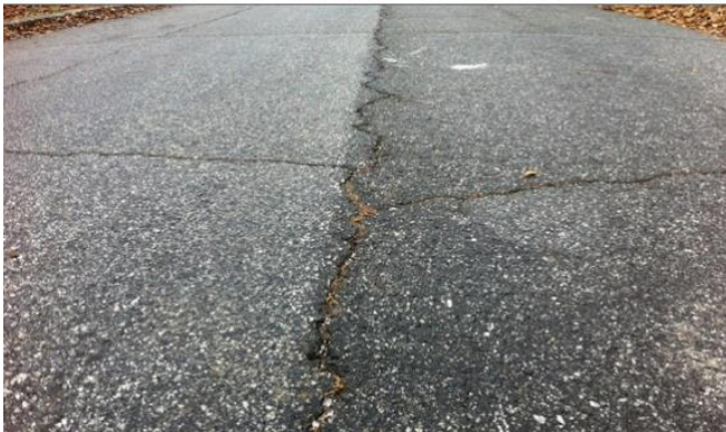
Longitudinal, Transverse, and Alligator Cracks
